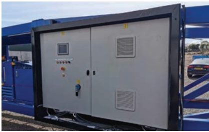
Tier 3 / Tier 4 Final Diesel Genset - 150Kva
