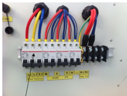
Main grid tied switch
